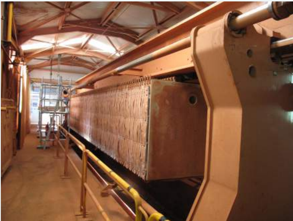
Filter press at Gardanne refinery
